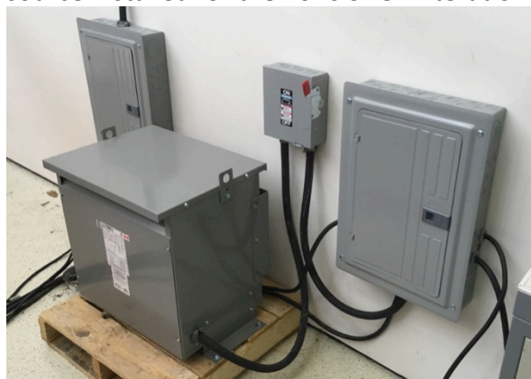
Fig. 20 Transformer and high-voltage power source installed for the 2016 SRGM iteration
