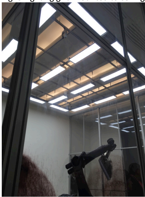
Fig. 8 Lighting grid mounted to ceiling
